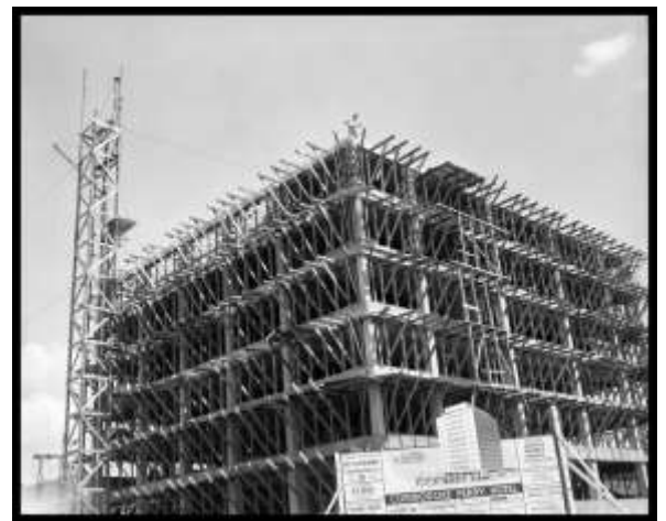
Construction of the Commodore Perry Hotel under in 1949 by Austin AGC leader Rex Kitchen's construction company
