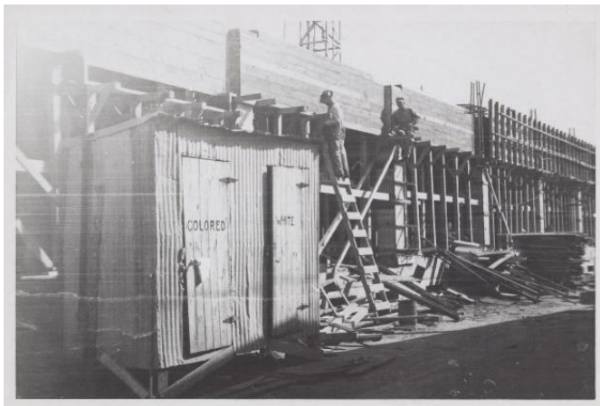
Workers building Calcasieu Lumber offices in downtown Austin circa 1946 (photo courtesy Austin History Center)
